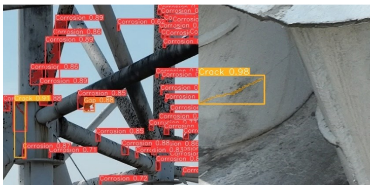
Fig. 2. Automatic detection of defects.
